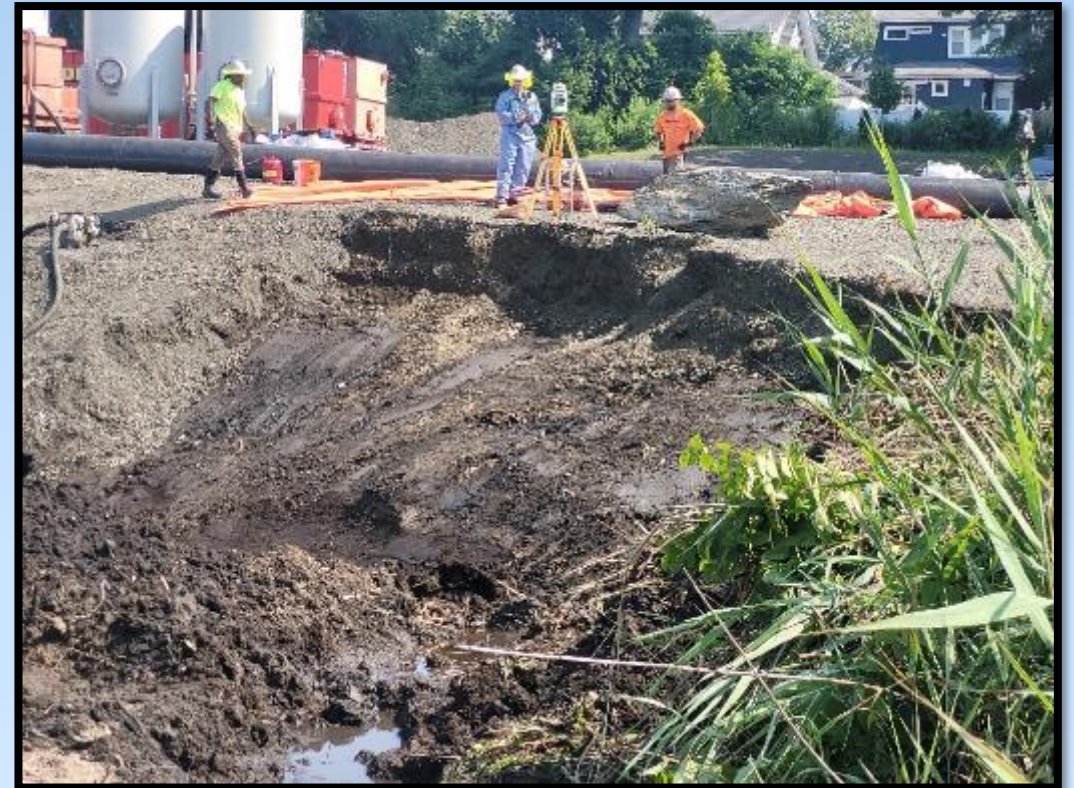
Bank Along Rear Vacant Lot
