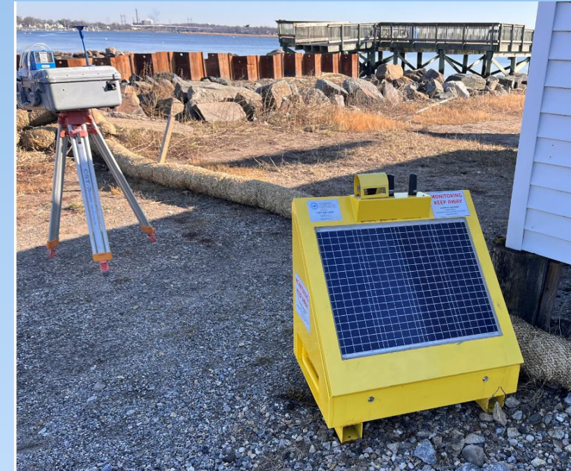
Dust and Vibration Monitoring Stations
