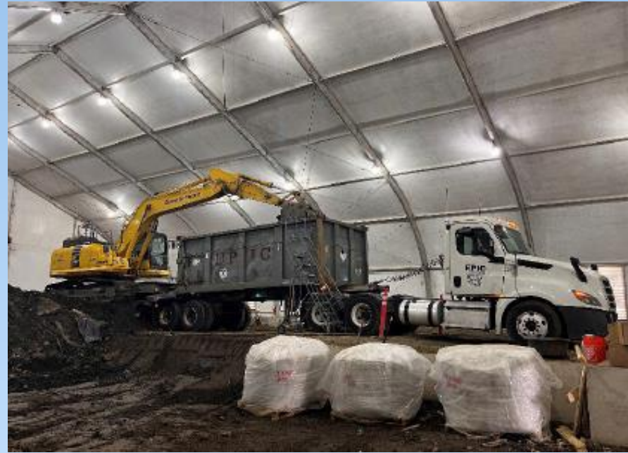
Loading treated PHC soil from Upper Ferry Creek into intermodal for off-site disposal at TFS.
