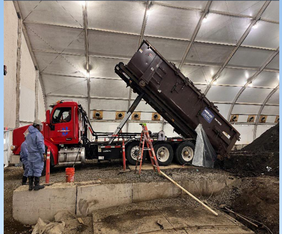
Material Drop to Material Handling Structure at OU4
