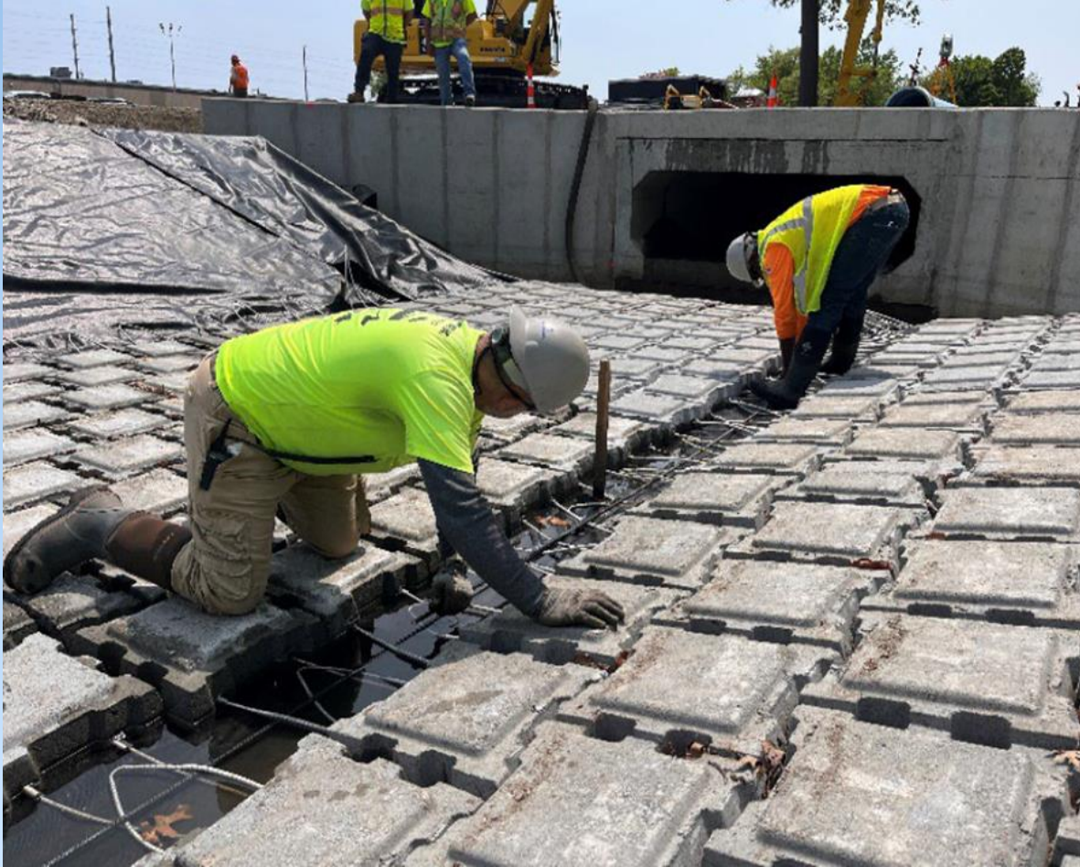
Articulating Concrete Block (ACB) Channel Armoring
