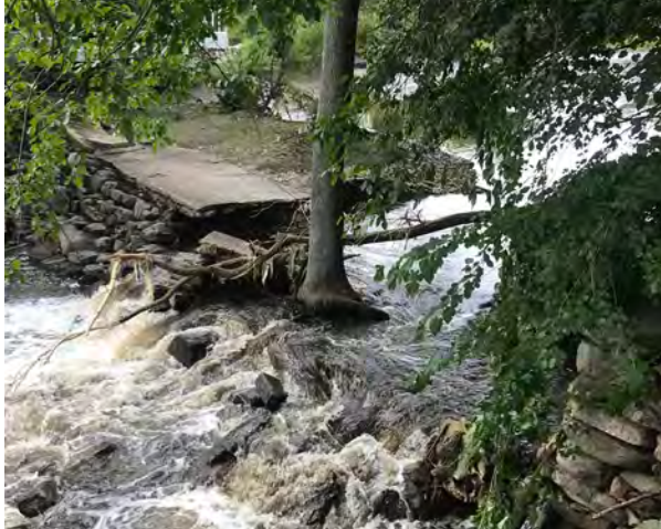
Minor Dam Washed Out along Sasco Brook. Photo by Brian Carey, Town of Fairfield
