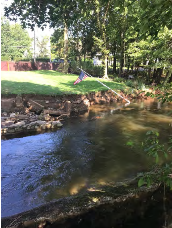
Bank Erosion along Rooster River from September 25, 2018 Storm. Photo by Town of Fairfield
