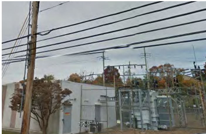
Lifeline Facilities: Electricity Transmission Baird Electric Substation (Credit: Google Earth 11/2015)
