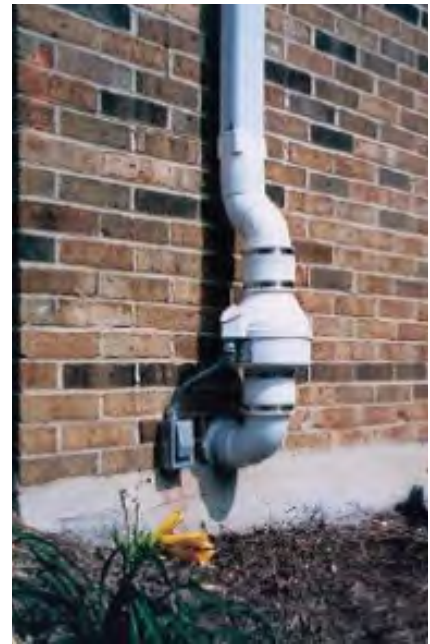
Image of Typical Fan and Vent Pipe in a Soil Vapor Mitigation System
