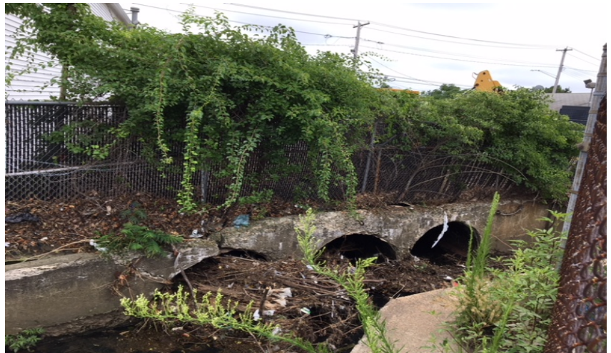
This photo of Bruce Brook shows a significantly damaged concrete headwall and clogged culvert pipes caused by debris.
